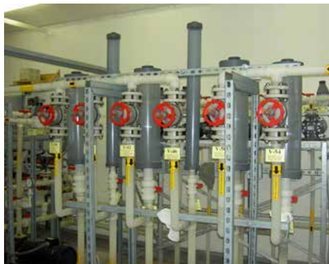
Figure 1: PVDF welded piping system in fluoride treatment facility.
