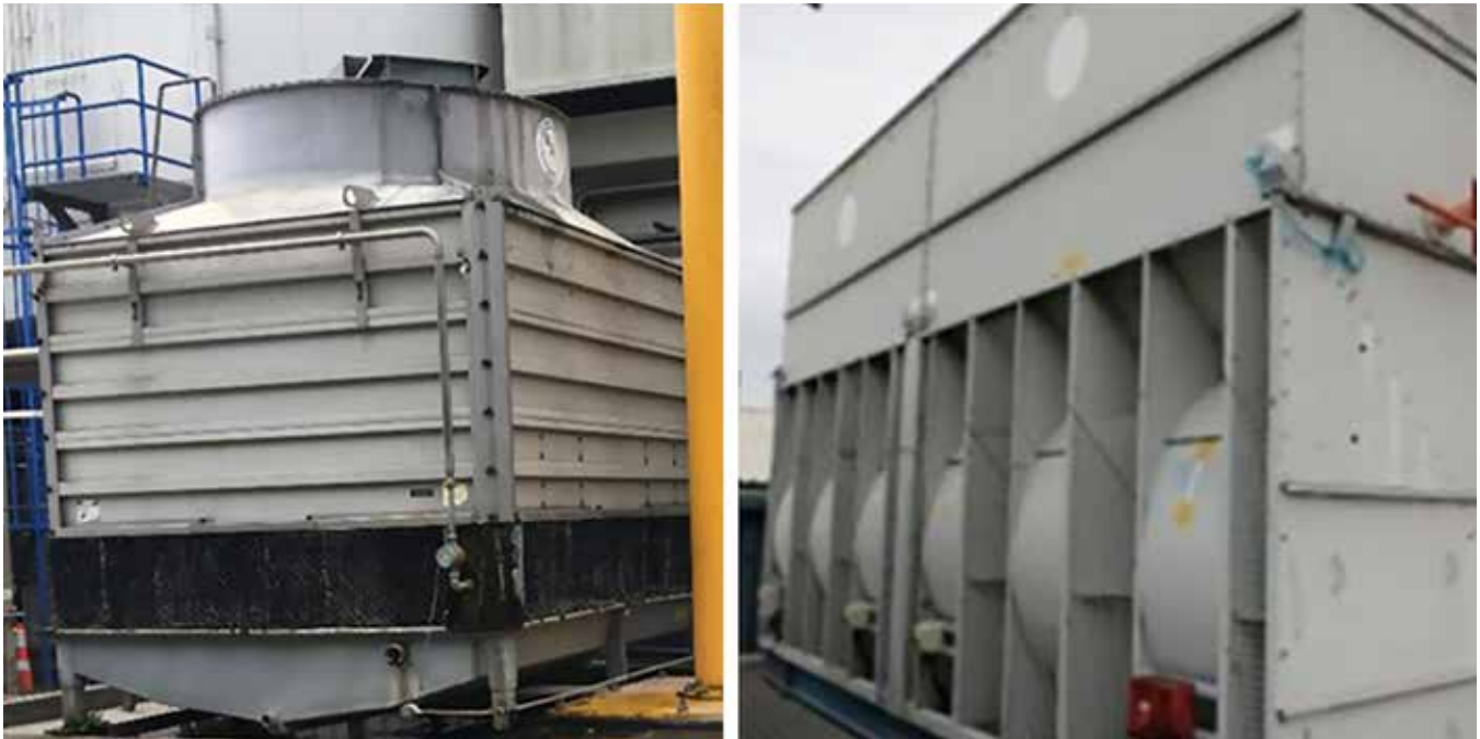
Figure 1: System 1—counterflow cooling tower (left); System 2—evaporative condenser (right).
